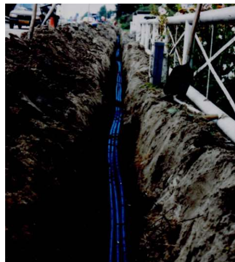
Figure 3. Open trench with undulating ducts
